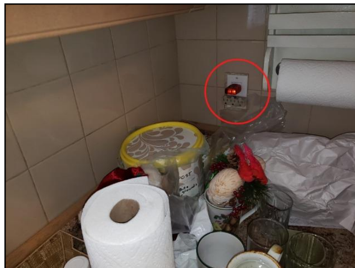
27. GFCI/GFI needed (Ground Fault Circuit...
