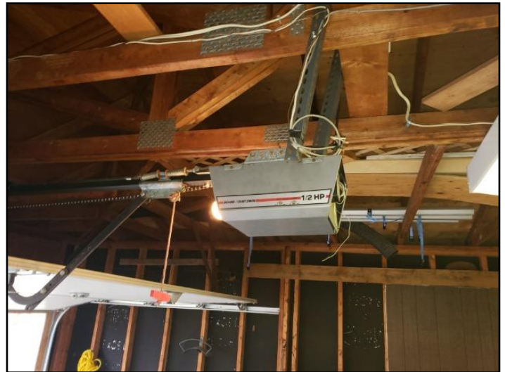
15. Sensors poorly located
