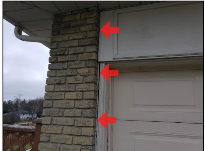
9. Caulking missing or deteriorated
