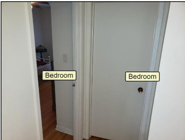
48. Loose or poor fit
