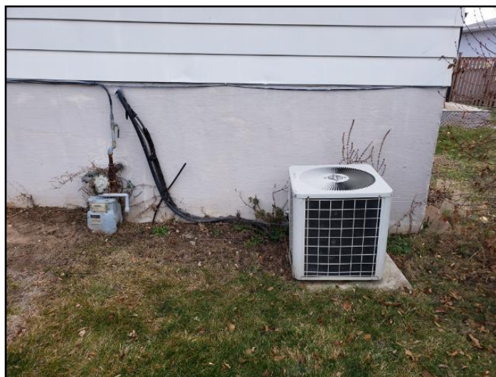
40. Missing electrical shutoff
