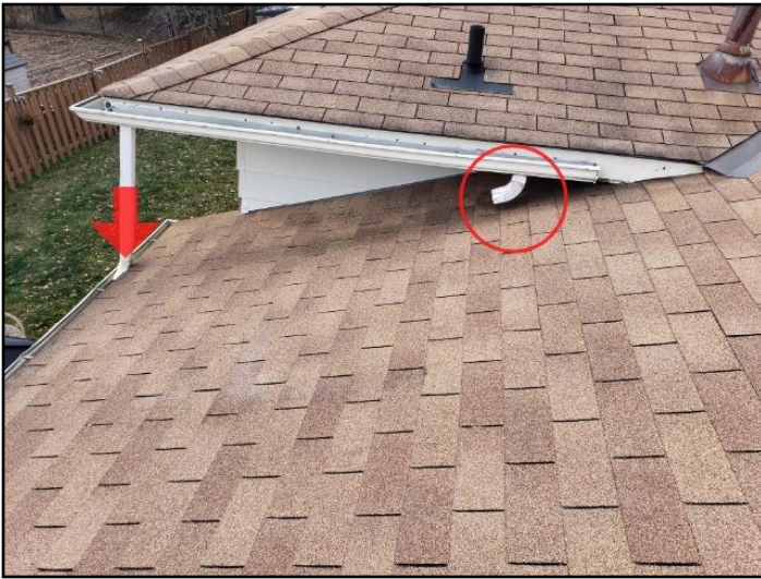
6. Discharge onto roofs
