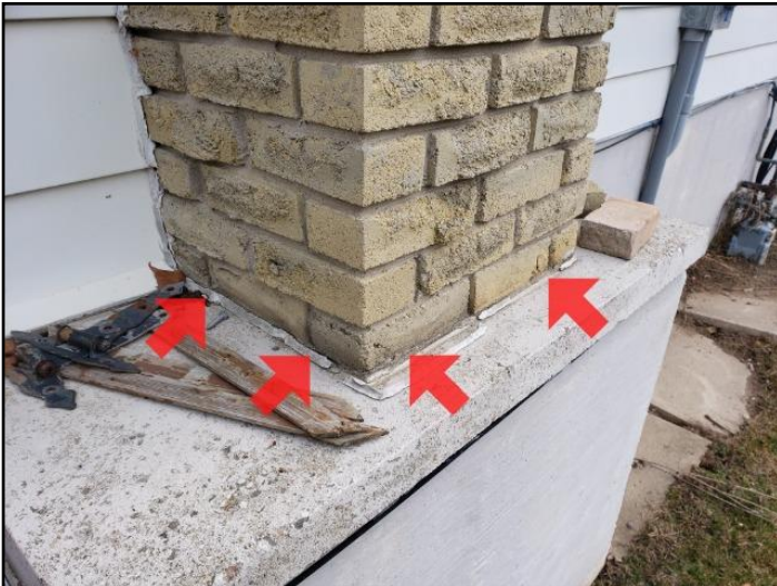
8. Caulking missing or deteriorated
