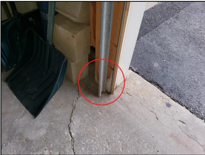
14. Sensors poorly located
