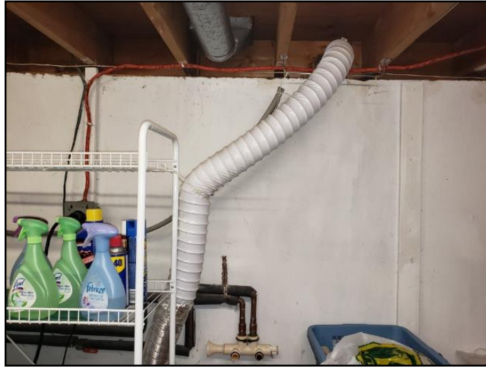
53. Plastic dryer vent
