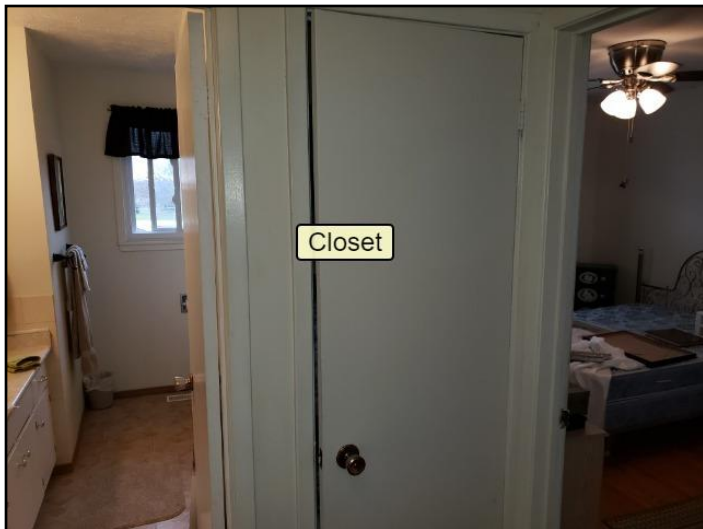
49. Loose or poor fit
