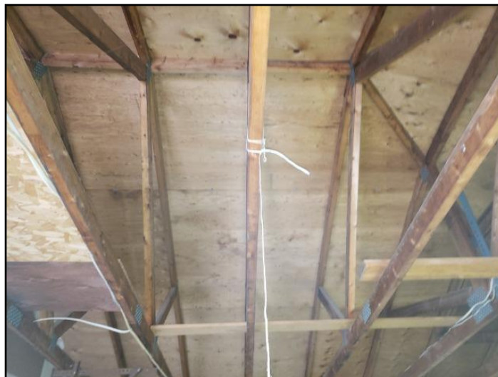
1. Garage roof not vented - Recommend adding a...
