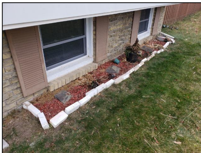
10. Too close to grade
