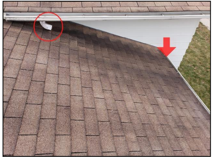
7. Discharge onto roofs
