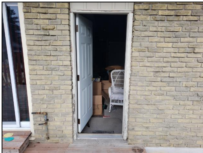
12. Paint or stain needed
