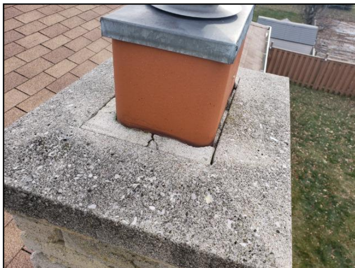
38. Open Seams - Recommend sealing the seams at...
