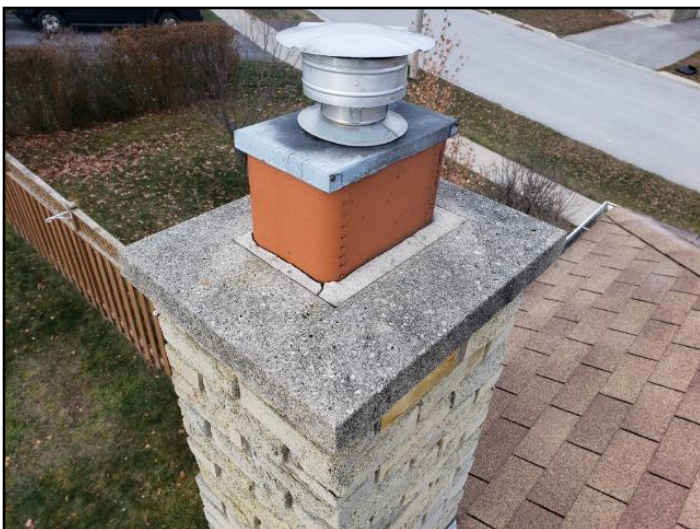
37. Open Seams - Recommend sealing the seams at...
